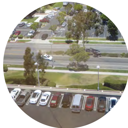
Upper Parking Deck in Need of Repair
