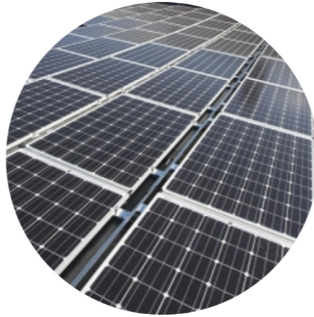
Desire to Increase Onsite Renewable Energy
